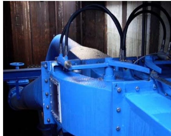
Figure 3: The Venturi at Waterboard Hunze & Aa's.
