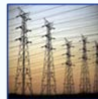
3. Power Sector Energy Efficiency
