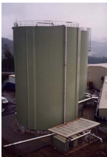
Figure 12 Digestion plant for bio-waste
