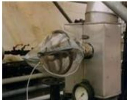
Figure 3.38: Bagging of a leaking valve
