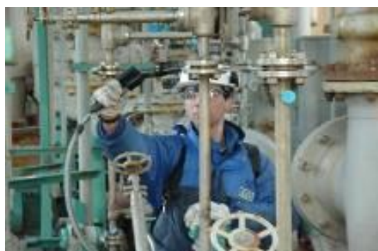
Figure 3.37: Leak concentration measurement
