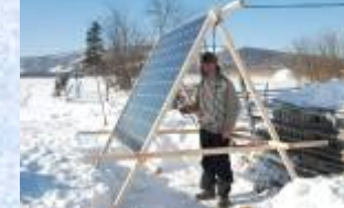
On the territory of a former farmstead Kashela the BR's supporting base with the aboriginal bee apiary is being built. For ensuring everyday life in the settlement solar batteries were installed
