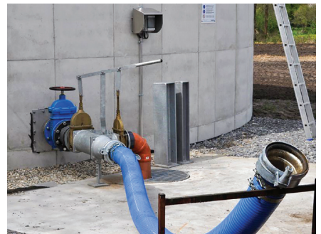
Fig. 8: Liquid manure drainage station with adjacent pit
