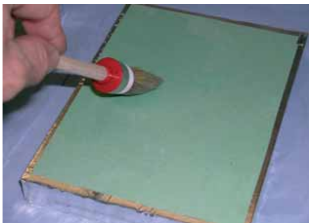
Fig. 7: Application by brush of a primer on plasterboard, the edges of the plasterboard sample are covered with a self adhesive aluminium foil.
