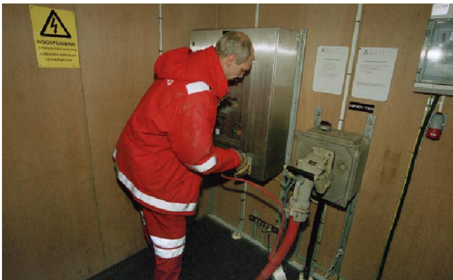
Picture 35: Supply of electricity for ships by means of a cable connection in port
