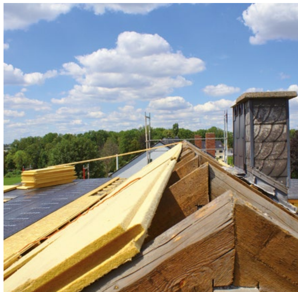
The insulation of roofs and façades as part of energetic refurbishment also improves summer heat protection. (Photo: © Marco Becker / stock.adobe.com)
