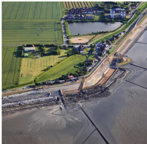
The dykes were reinforced at the Alte Koog on Nordstrand in Schleswig-Holstein. By 2016 the first 'Klimadeich' was installed here. (Photo: © Lehnerfoto / Generalplan Küstenschutz SH 2022)
