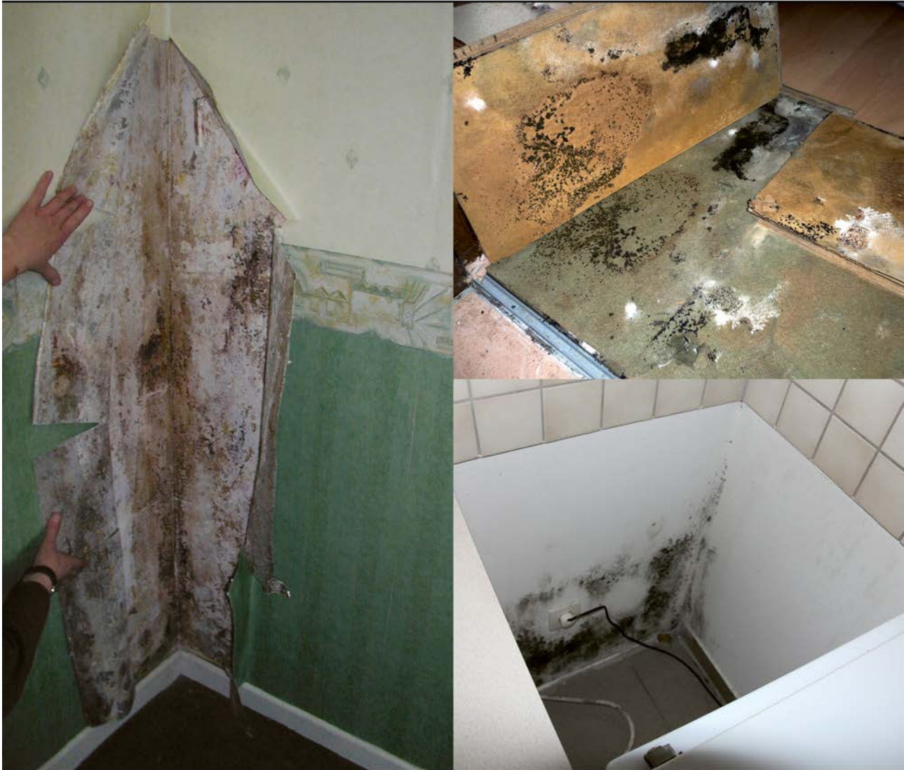
Source: left: Lorenz, Institute for Indoor Diagnosis; right: Betz, Experts Office for Building and Interior Analysis
