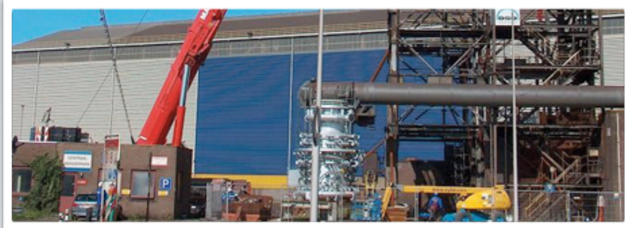
HiSarna Blast Furnace (Tata Steel)
