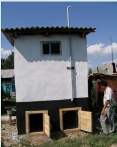
Double vault UDDT. Faeces chamber doors are opened for demonstration. The ventilation pipe seen here has too small a diameter and was replaced later.
