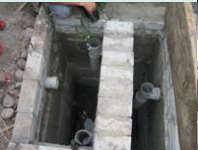
Sedimentation tanks of Ivanovka constructed wetland.
