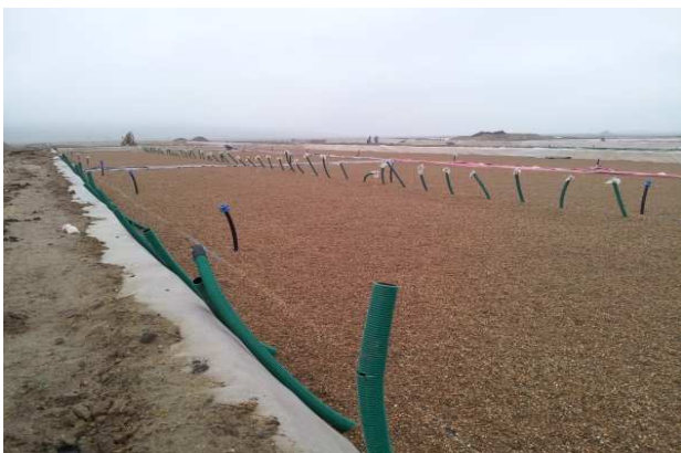
Photo 1: Orhei Constructed Wetland Treatment Plant
