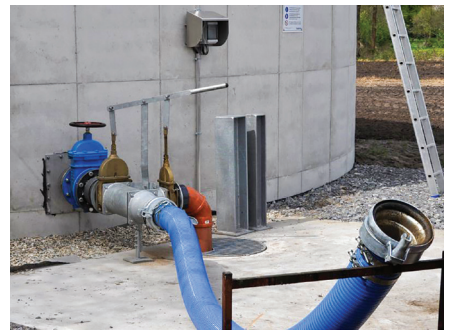
Fig. 8: Liquid manure drainage station with adjacent pit
