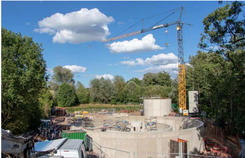
New Erfweiler-Ehlingen sewage treatment plant
